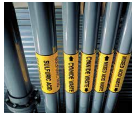
Installed piping for the transport of chemical substances
